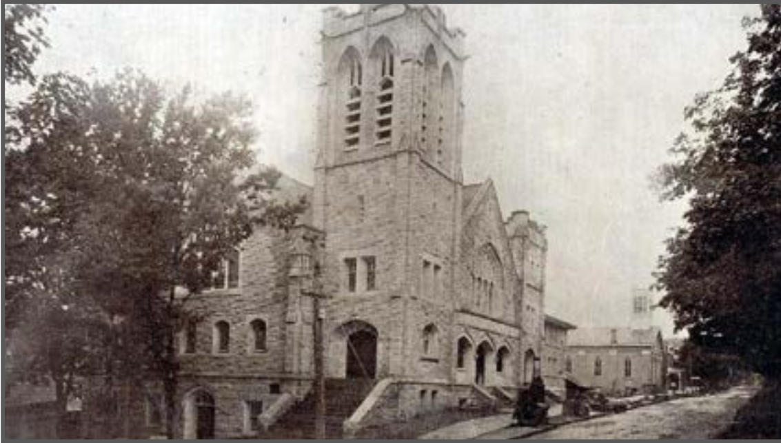
This c. 1912 photo shows the church still under construction; the former U. P. Church appears in the background
