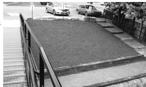
East section of exhibit area with newly installed terrace, brick walkway and mulch — ready for planting.
