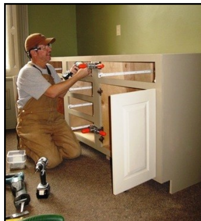
Bill Crain recently completed his project of new custom built cabinetry for the Living on the Land Learning Center
